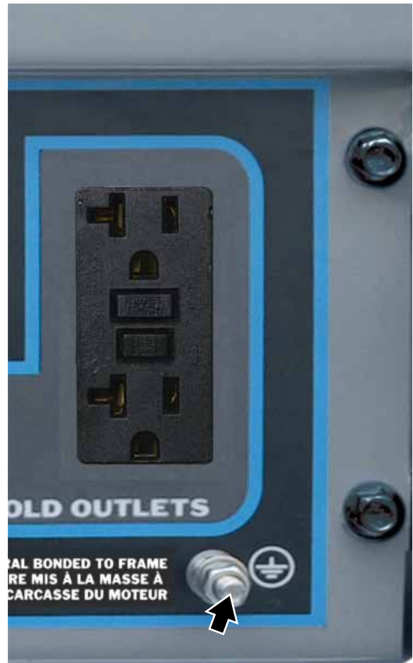
Figure 12 – Ground Terminal on the Control Panel
