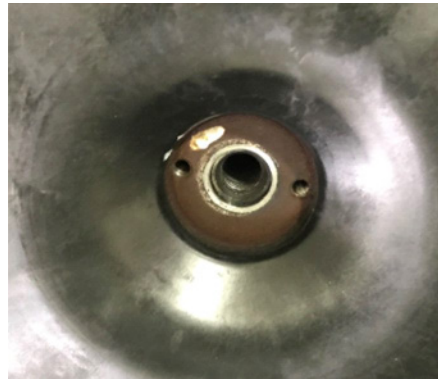
FIGURE 62. FAN HUB AND END OF ROTOR
