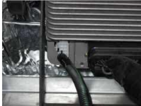
Figure 2.2 - Harness installed to Controller.
