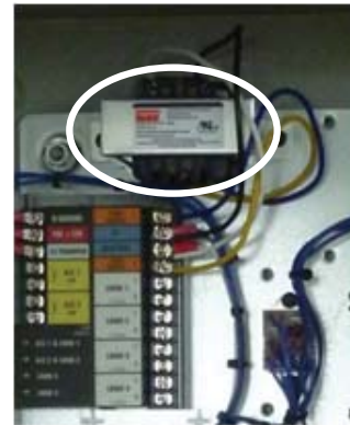
RTSR TRANSFORMER MOUNTING
